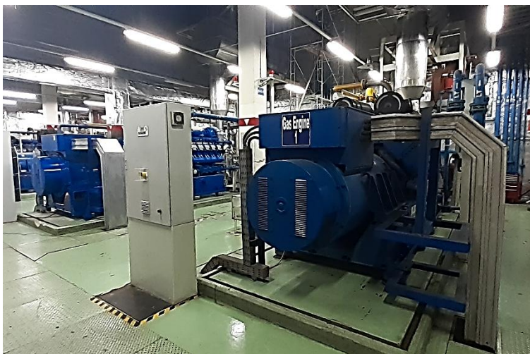
MWM TCG 2020V16K Gas Genset
