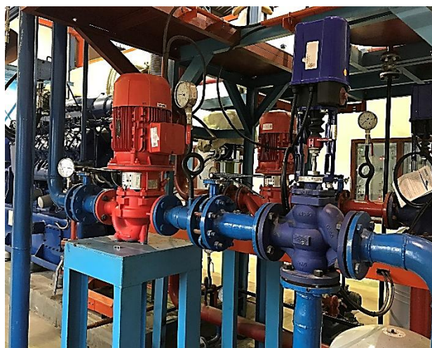
Gas Genset Auxiliary Piping
